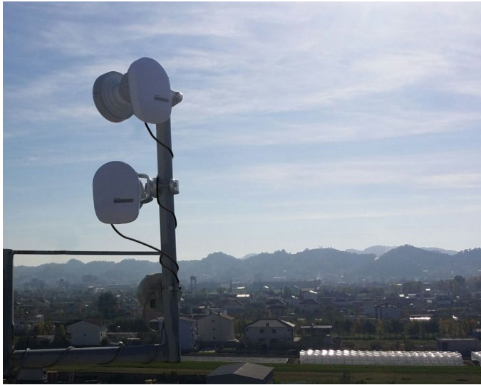
Co-location with RF elements® Symmetrical Horn Antennas in Albania
